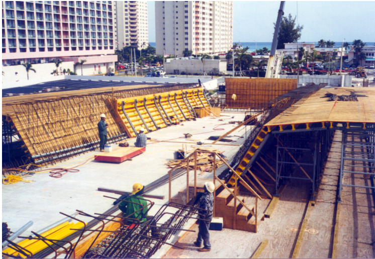
Figure 1.19 – Web and Cantilever Wing Formwork for a Single-Cell Box Girder
