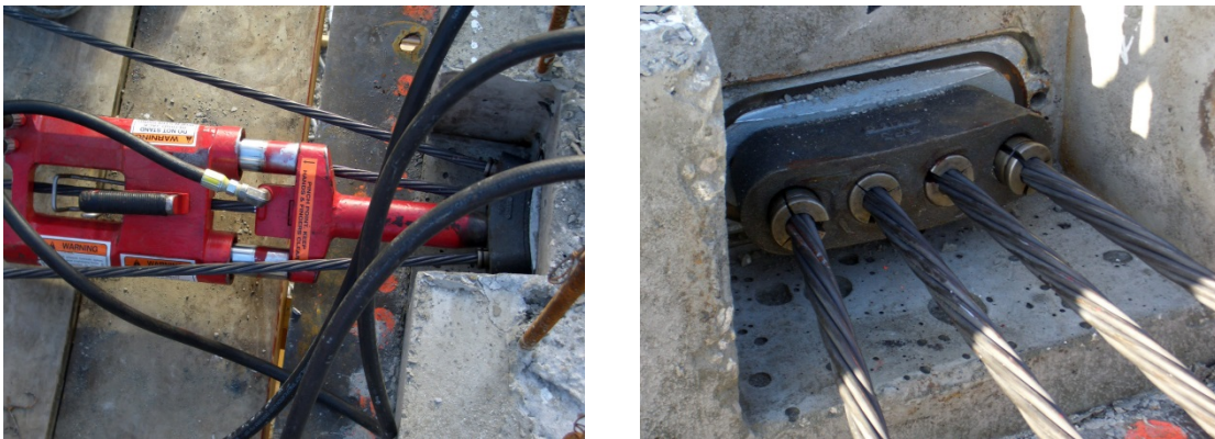
Figure 8.38 – Mono-Strand Stressing of a 4 Strand Tendon (left) and Anchorage After Stressing 2 nd Strand (right)
