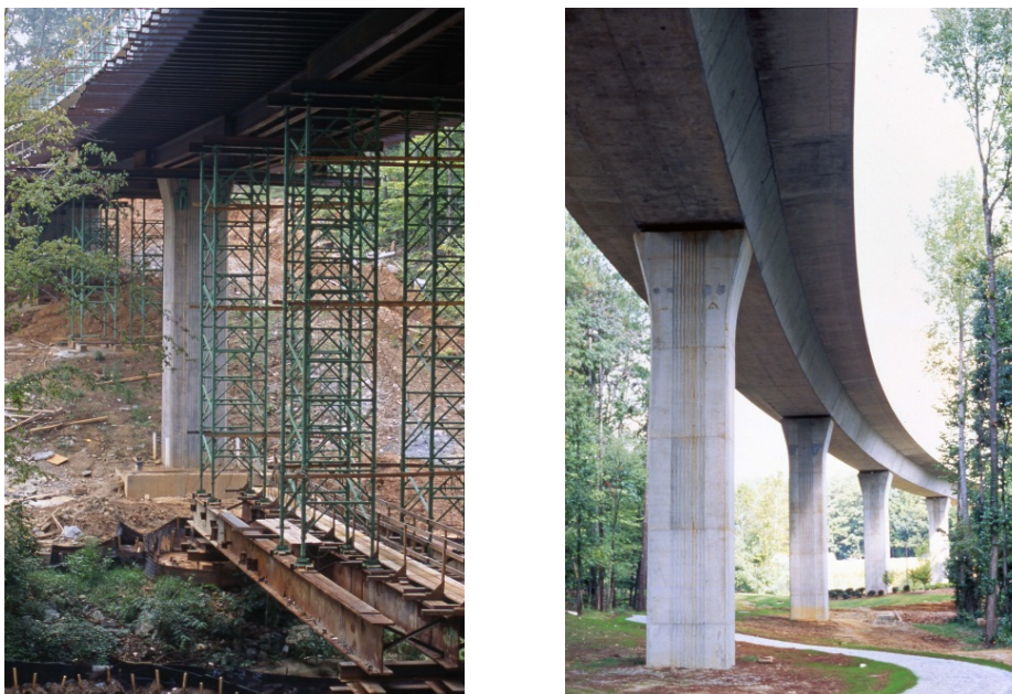
Figure 1.1 – Cast-in-Place Post-Tensioned Box Girder Bridge for the Metropolitan Atlanta Regional Transit Agency (MARTA) – under construction (left), completed (right)
