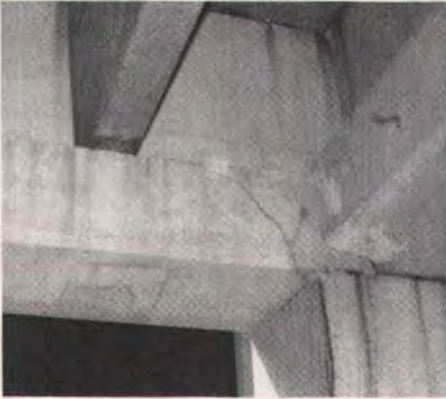
Fig. 5. Beam ledge end corbel failure (applied loads and reaction in alignment).
