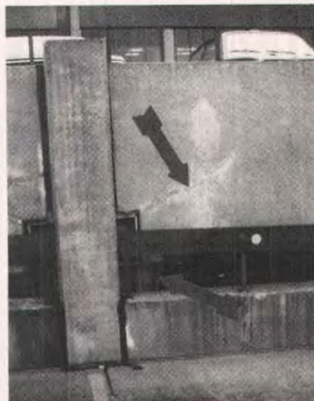
Fig. 8. End support dap distress caused by insufficient dap and torsion reinforcement (upper arrow indicates epoxied dap cracks and lower arrow points to modified end support).
