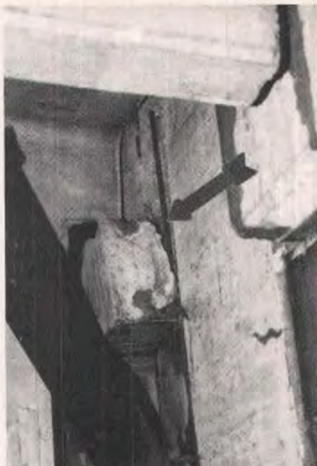
Fig. 7. Ledge failure near beam end.
