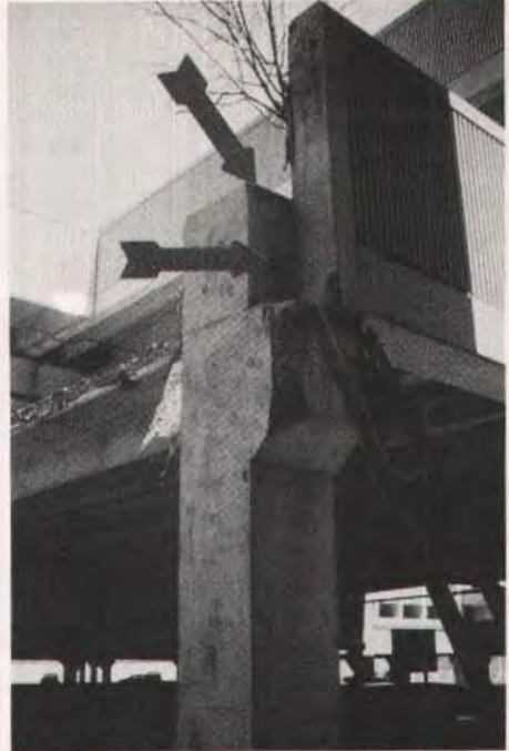
Fig. 6a. Overall view of torsion equilibrium tension insert connection (top arrow indicates bearing pad location and lower arrow points to failed tension insert).
