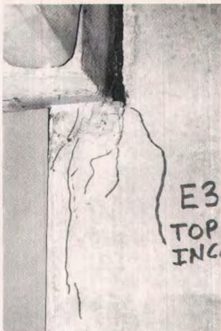
Fig. 3b. Close-up of typical bearing distress.
