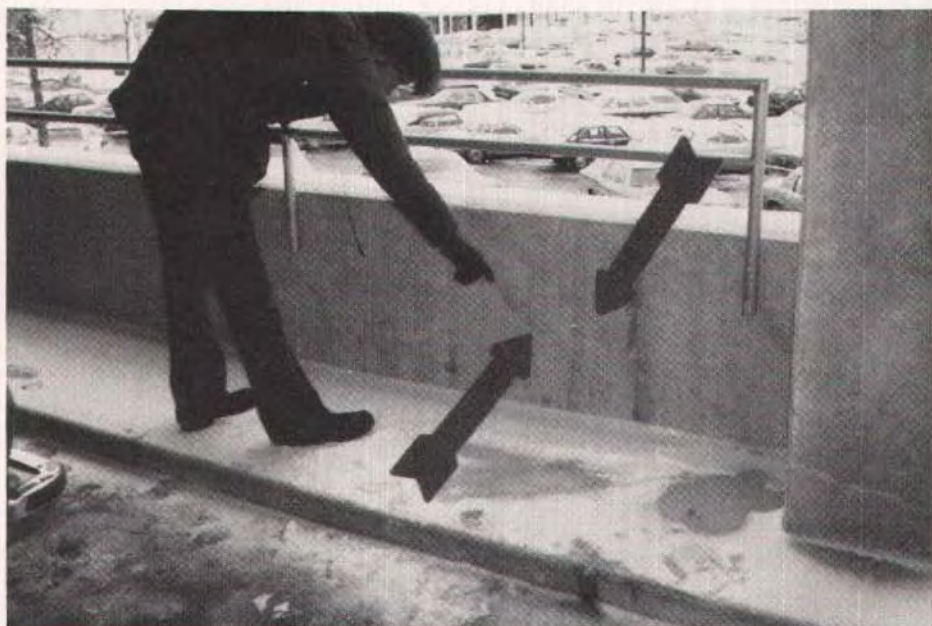
Fig. 2b. Top view of end cracks (arrows).
