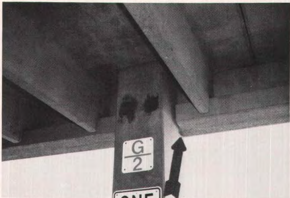
Fig. 2a. Underside view of beam end torsion cracking within distance "d" caused by equilibrium connections and internal torsion (arrow indicates location of reaction).
