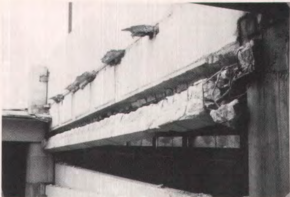
Fig. 9. Complete separation failure of ledge from beam web.
