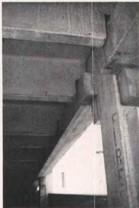
Fig. 1a. Lack of overall torsion equilibrium: underside view showing non-alignment of applied loads and end reaction.
