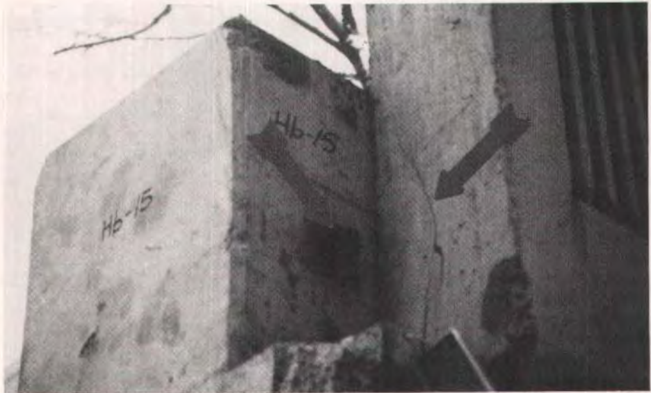
Fig. 6b. Close-up view of failure (left arrow points to insert and right arrow indicates shear cone crack failure plane).
