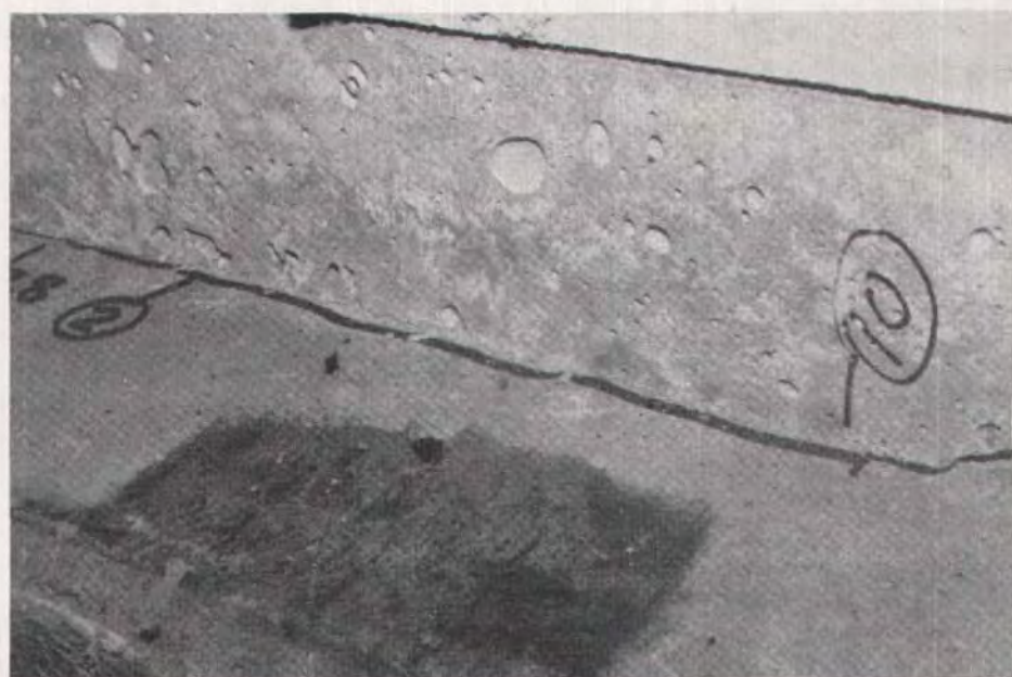
Fig. 20. Crack at ledge/web junction (Specimen 2).
